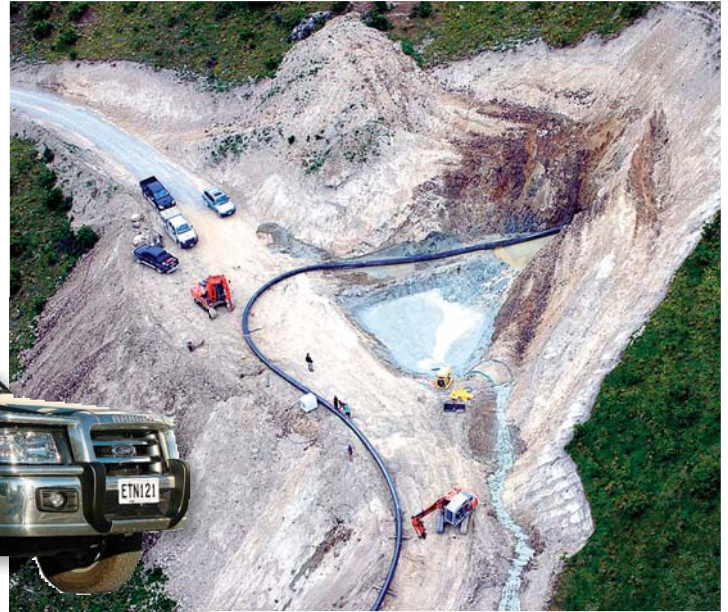
Directional drilling a 600mm diameter hole over 200 metres through a solid rock hill in Omarama, then installing a 450mm diameter PE irrigation pipe
