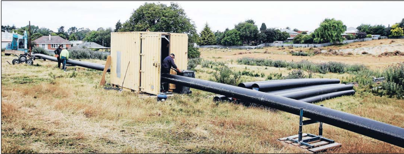
Pipe preparation: Sections of the new Gardens Gully sewer renewal pipe are being welded together ready for installation.
