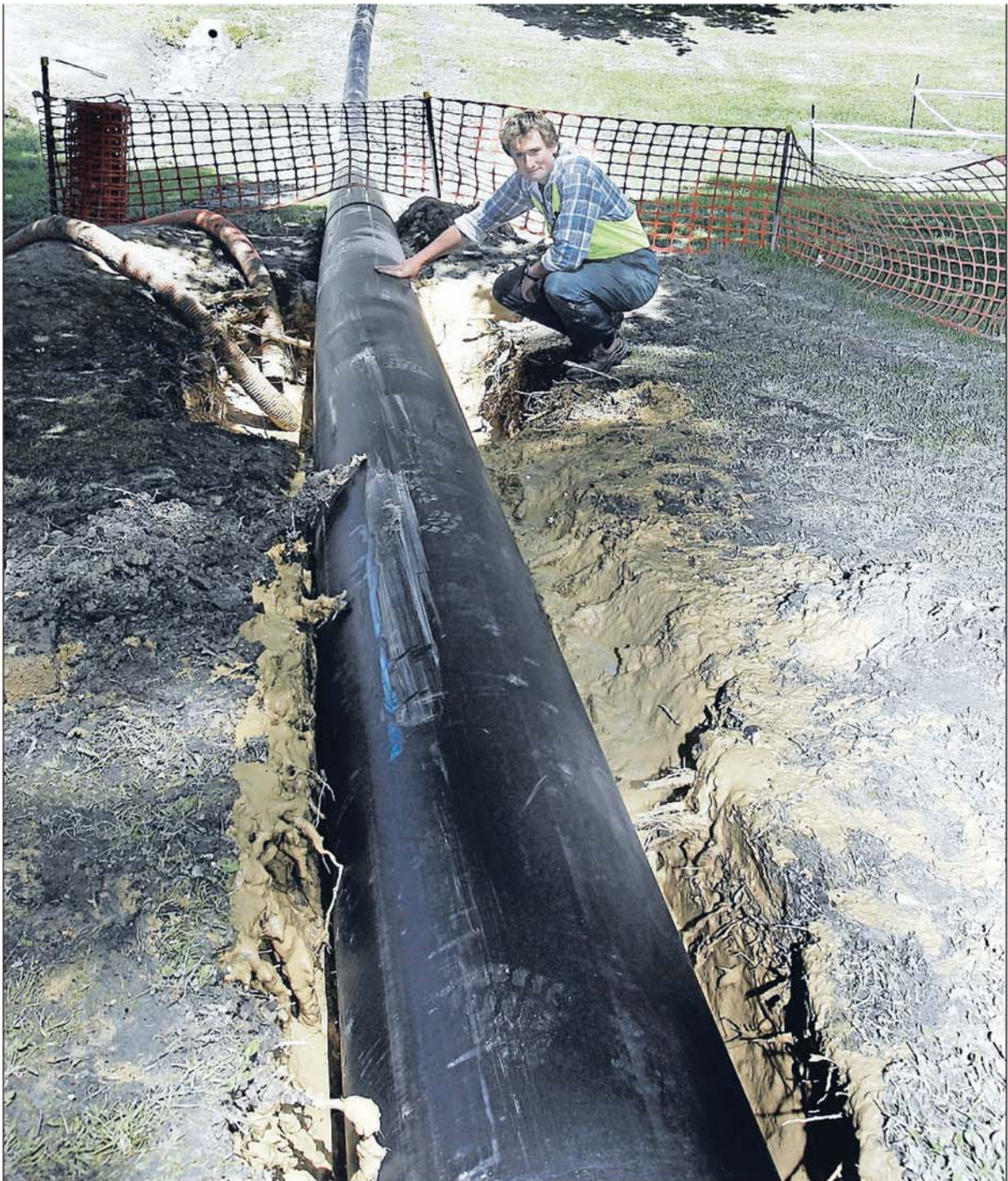
Stormwater solutions: Hadlee and Brunton director David Brunton surveys the new stormwater pipe that will run between West End Park and Sealy St.
