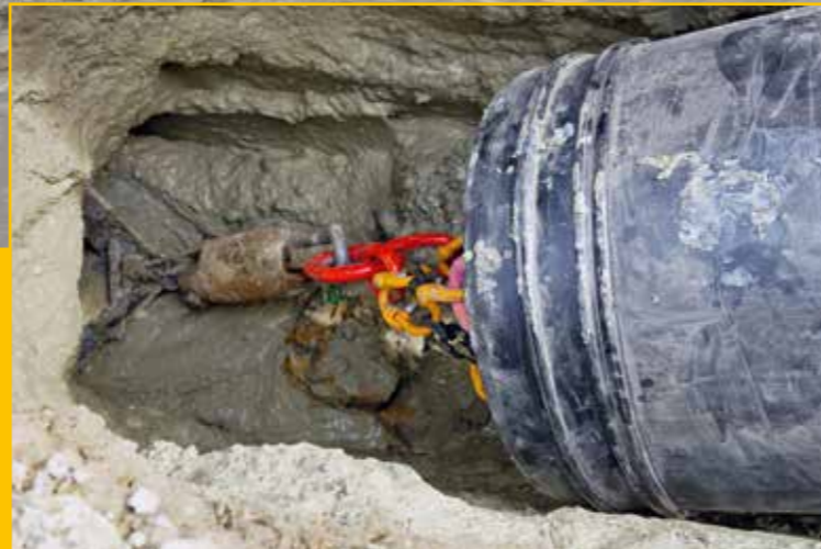
Preparing to pull a length of pipe through an already-drilled hole. Because it minimises surface disruption, directional drilling works well in urban environments
